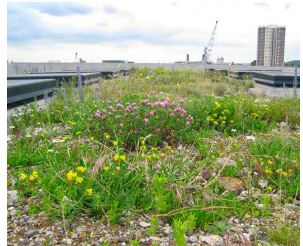
Self seeded brown roof - Laban data centre
